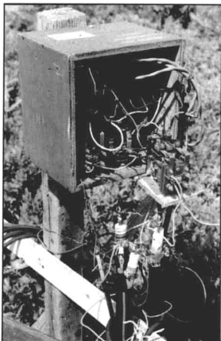
Antenna control with open-frame relays and no coax connectors.
